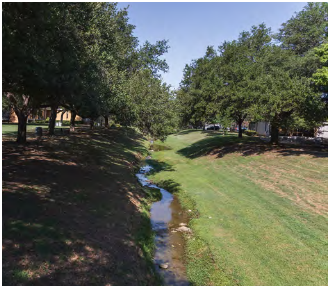
Non-natural creek edges lead to dangerous maintenance routines on steep slopes and increased erosion. Image by Mend Collaborative
