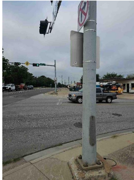
Figure 13 – Example of Missing Push Button
