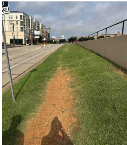
Figure 7 – Example of Sidewalk Gaps
