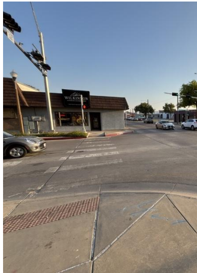
(A) Faded Crosswalk at S Bell Ave.
