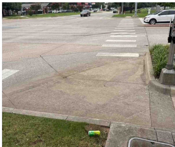
Figure 12 – Example of Faded Crosswalk Markings and a Non-Directional Curb Ramp
