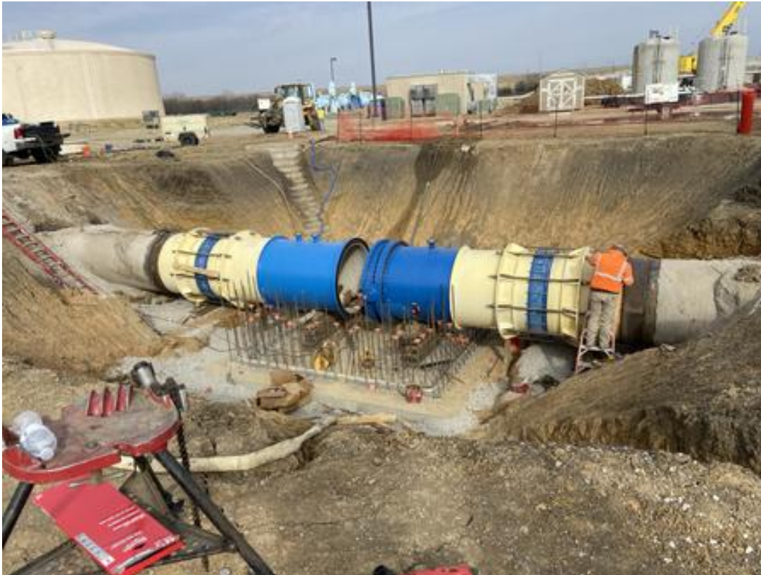
New 60" piping and valve
