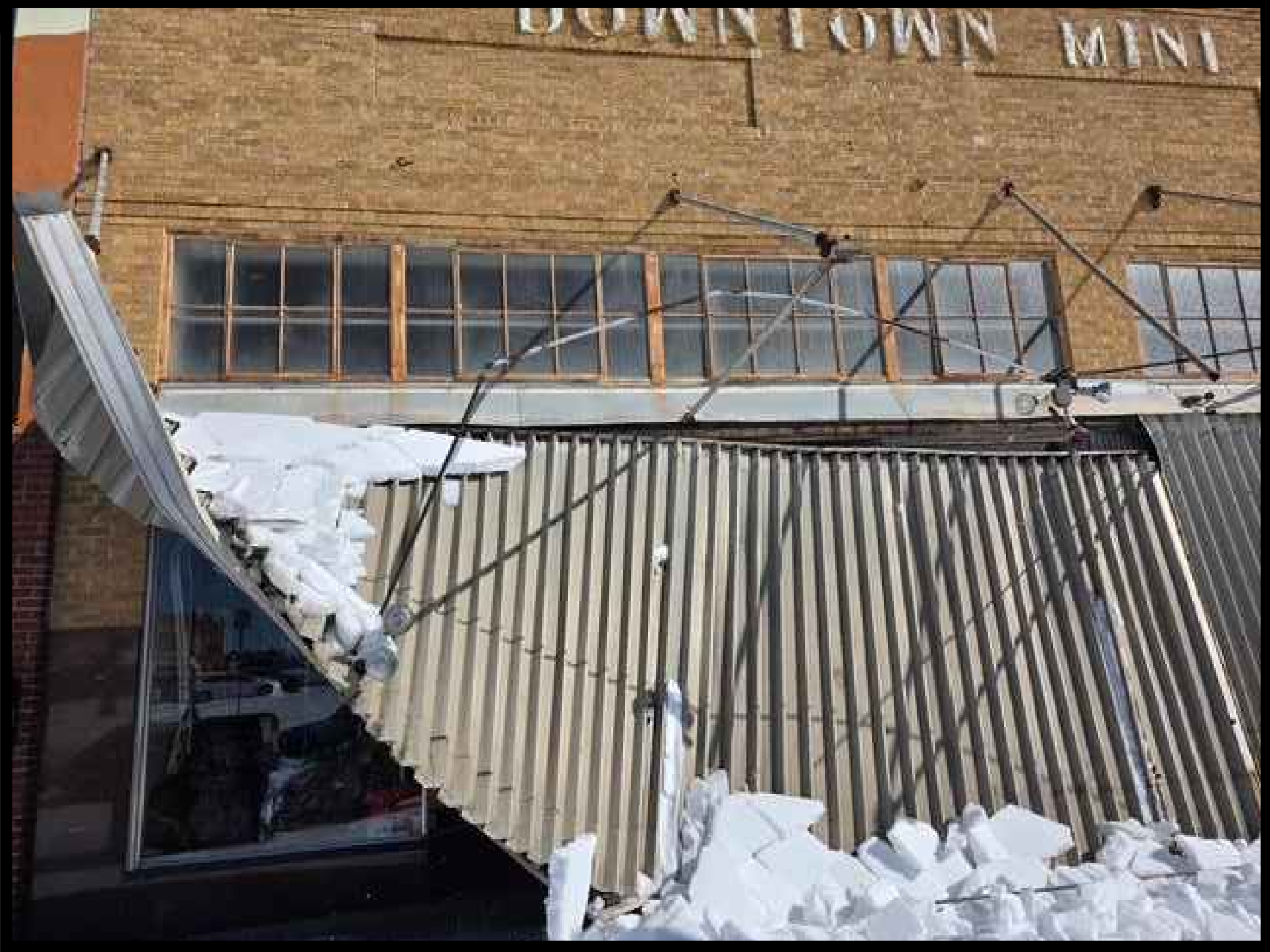
2 AWNING FAILURE NTS
