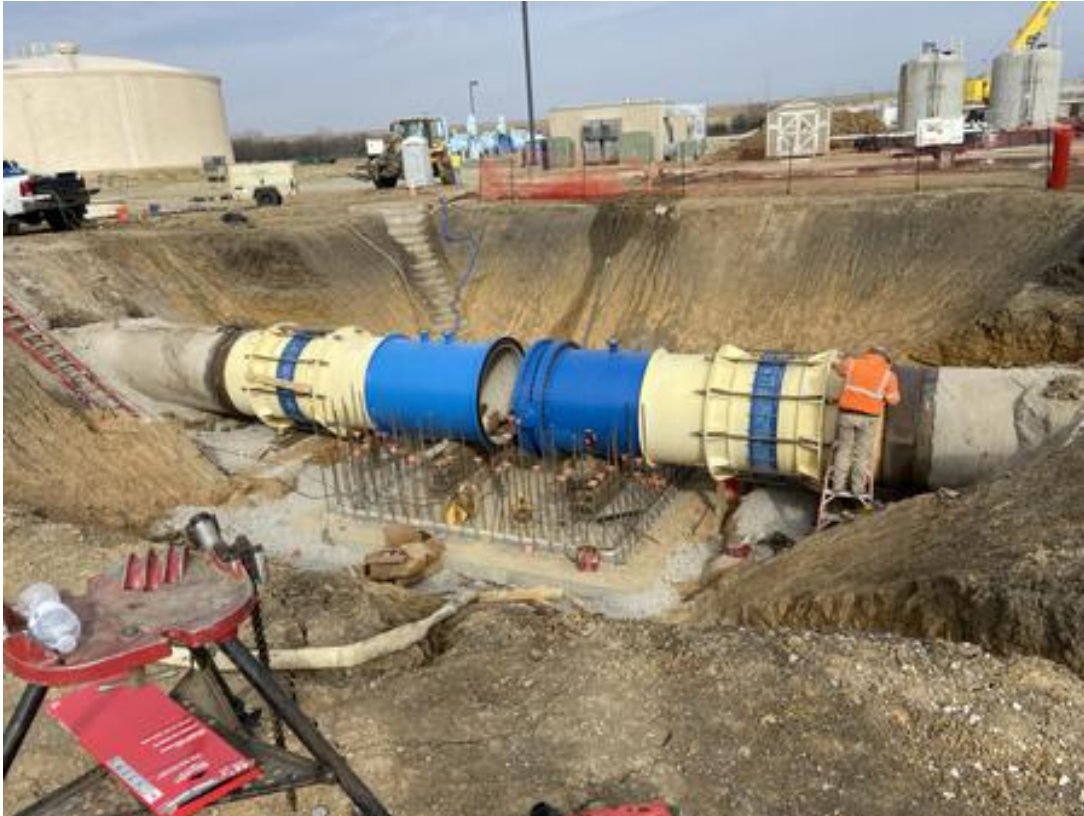
New 60" piping and valve
